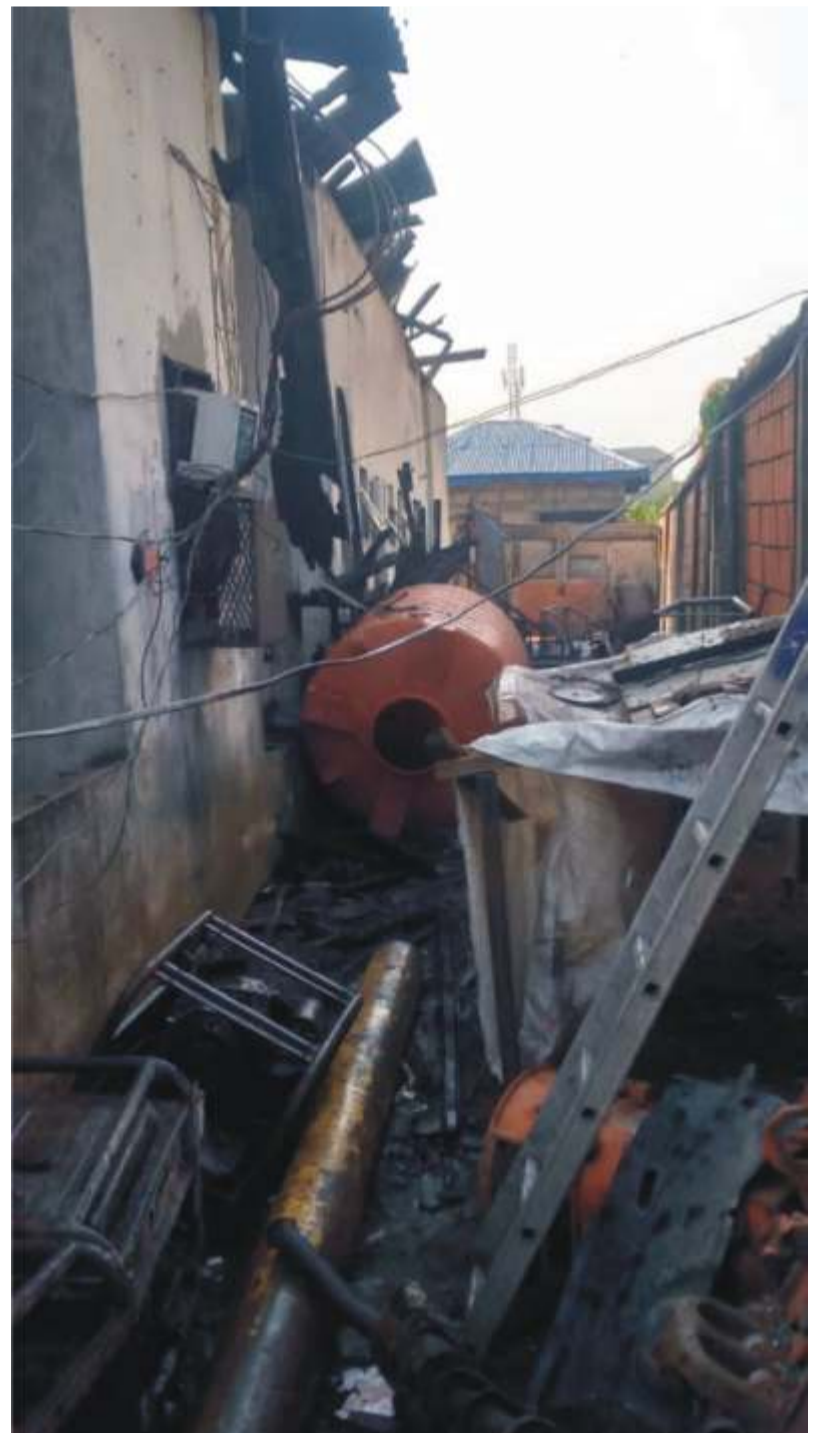
Side view of burnt police station
